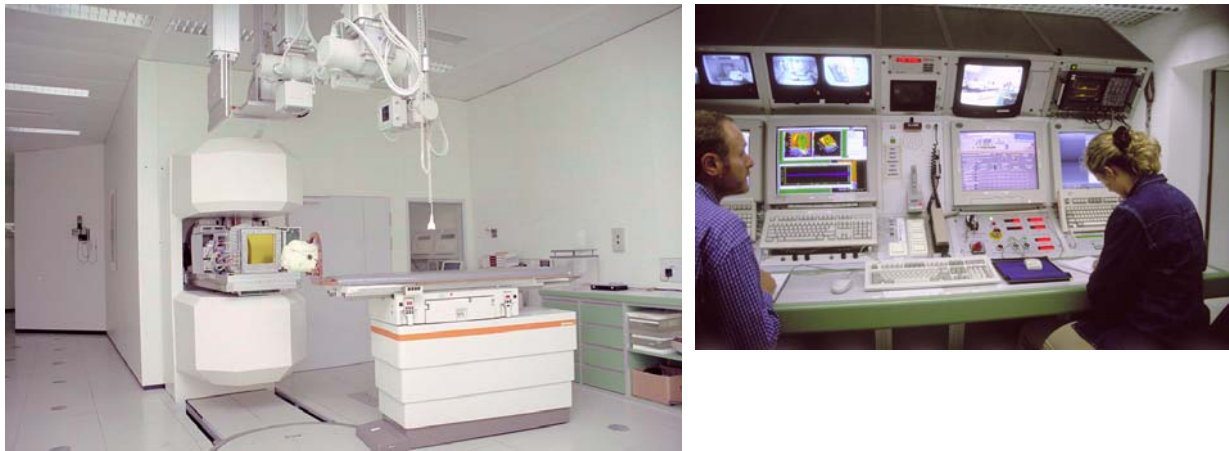
FIG.4. Treatment room and local control room of the GSI treatment unit.
